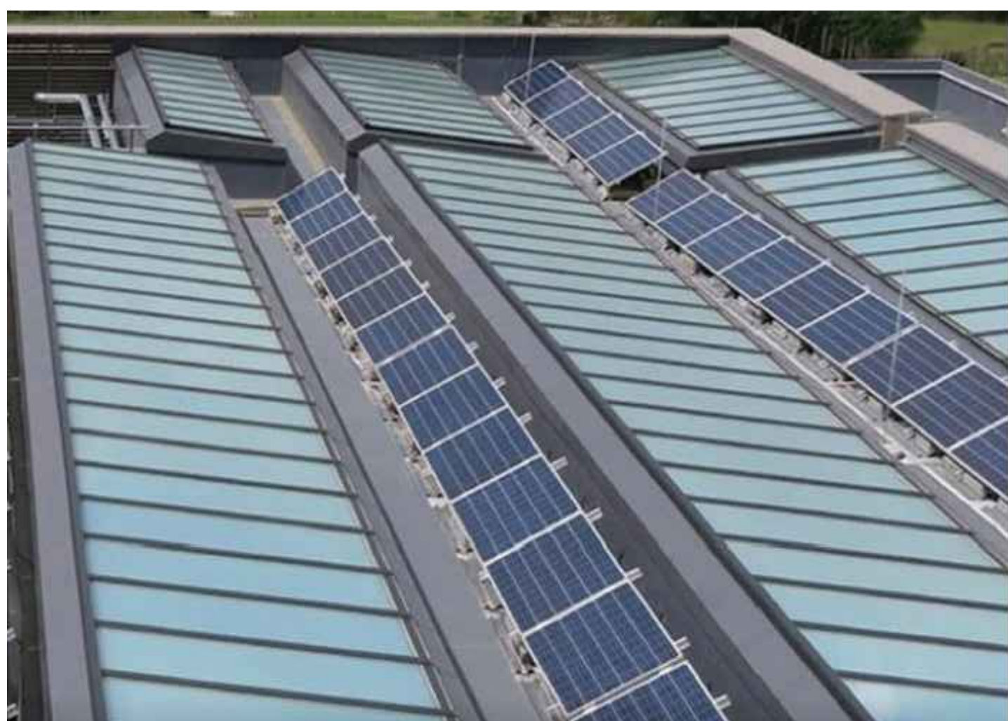
SKYLIGHT & SOLAR ROOF SYSTEM
