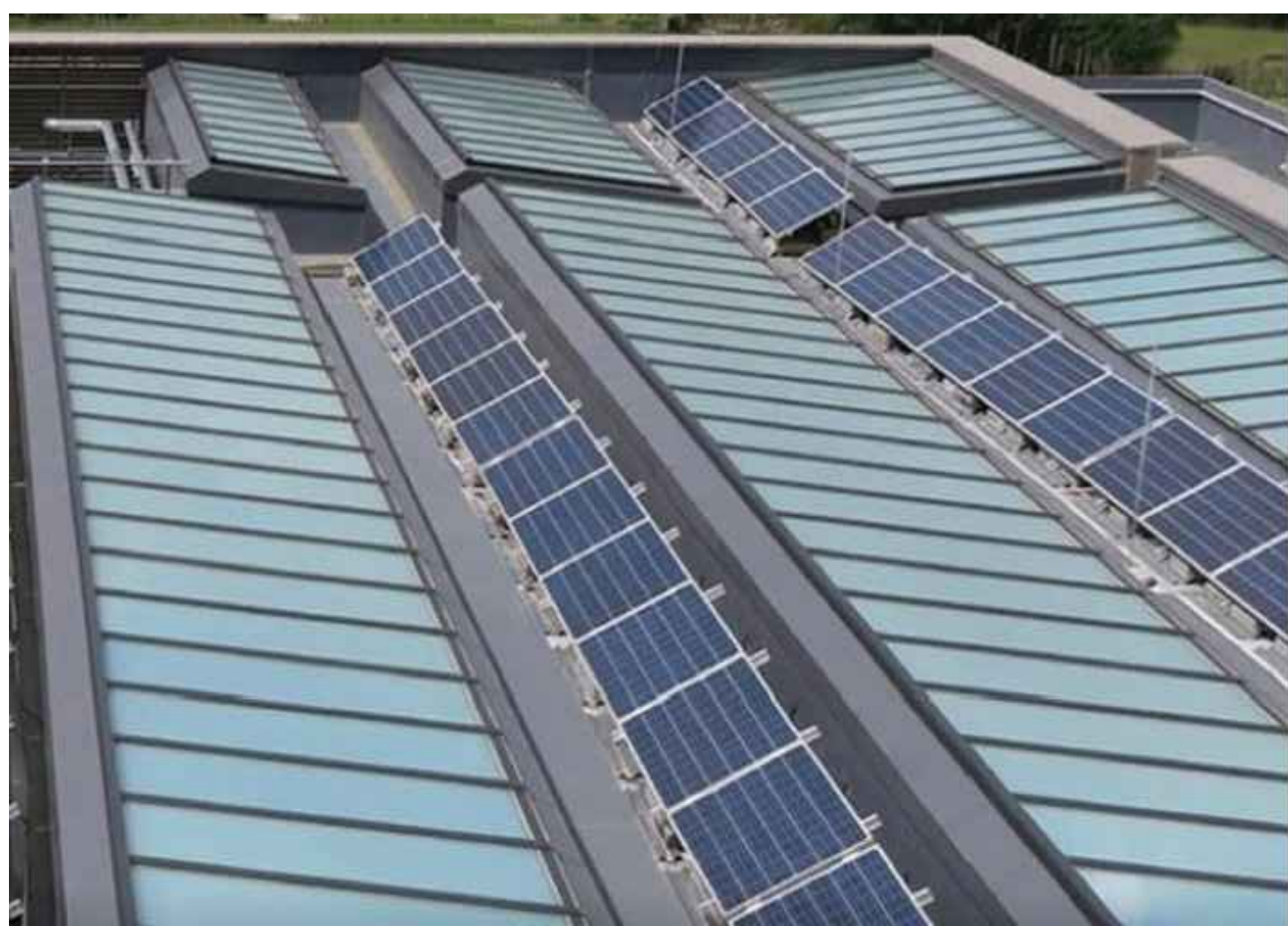
SKYLIGHT & SOLAR ROOF SYSTEM
